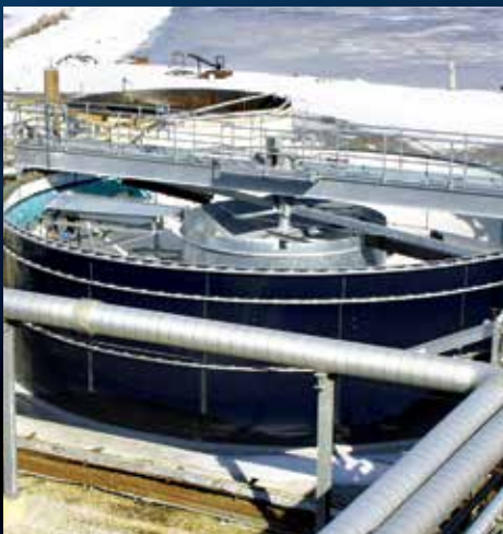
Wastewater Clarifier / Sludge / Storage / Mixing
